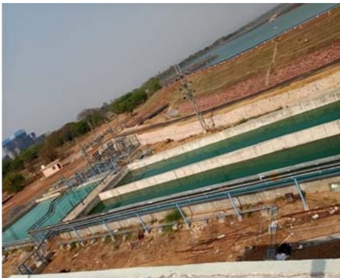
AWRS Plant at Odisha
