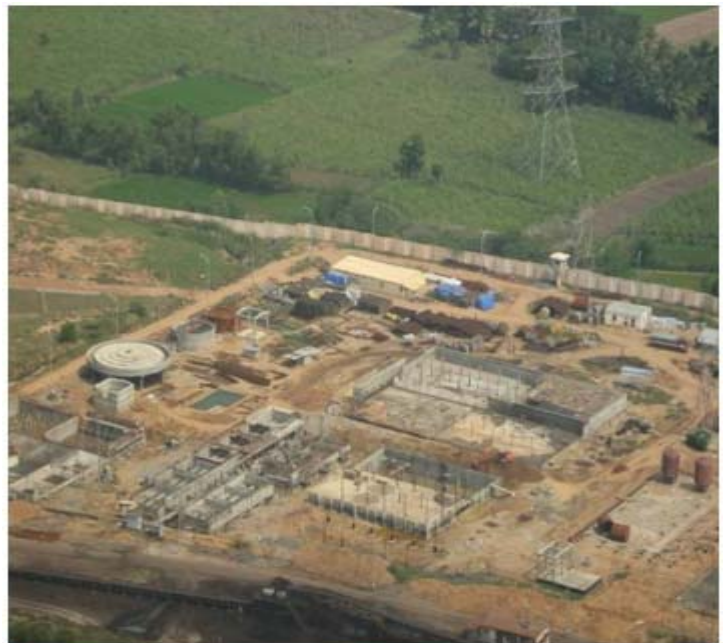
WTP & ETP FOR NEYVELI LIGNITE CORP. TAMILNADU
